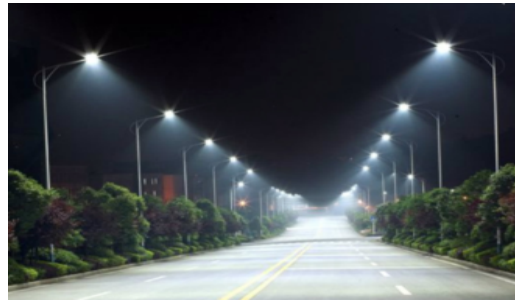
50,000 street lights and 6000 sign lights
